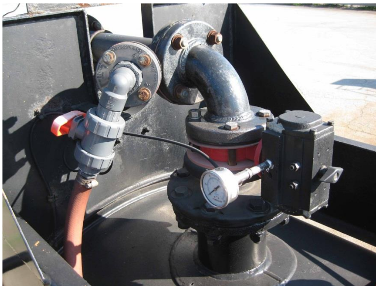
Miscellaneous in-line plumbing not protected.
