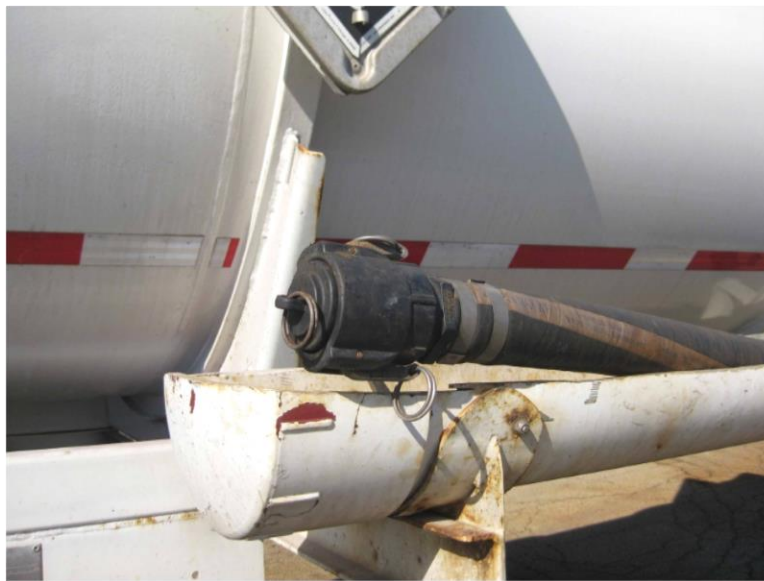
Off-loading hose not protected
