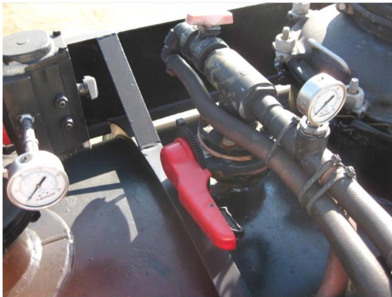
Miscellaneous in-line plumbing not protected.
