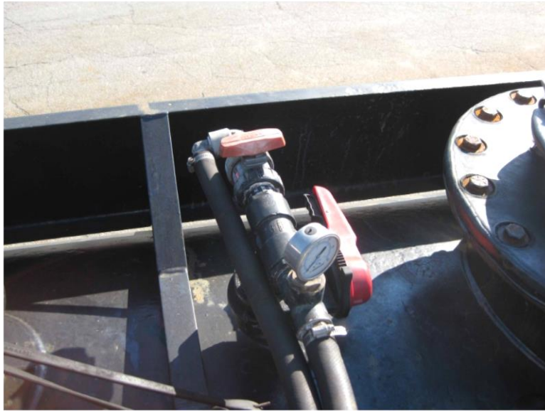
Miscellaneous in-line plumbing not protected.
