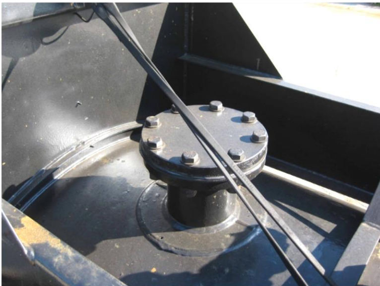
Torqued bolts not protected.
