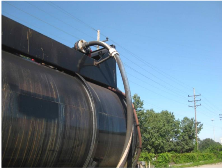
Miscellaneous in-line plumbing not protected.
